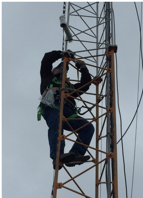
Attention to safety, with fall hazard equipment in place, in case of lost grip on cold trusses.
