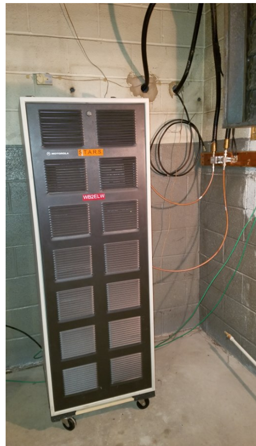
The New Colden Repeater
