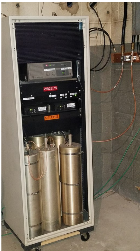
The New Colden Repeater
