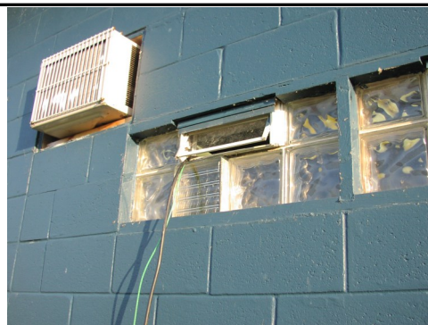
COAX AND GROUND CABLES, (NOT GENERATOR FEED LINES)
