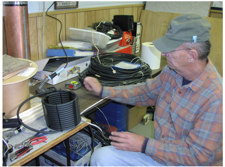
JON HALL, KC2QKB, PREPARES COIL FOR INSTALLATION BETWEEN ANTENNA AND FEED LINE
