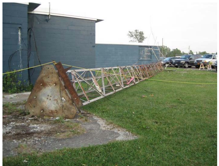
Another view of our downed tower.
